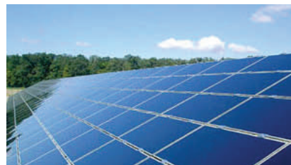
Photovoltaic Installation in Germany
